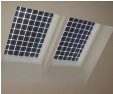
Interior Skylight View of Solar Panels
